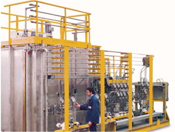
Corrosion inhibitor, Antifoam and Antiscaling Injection Package
